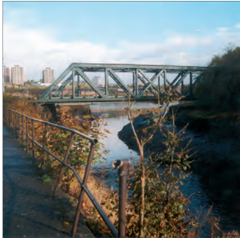
Landscape elements are in poor condition
