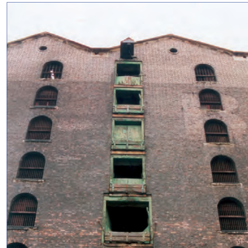
Derelict warehouses along Hanover Street
