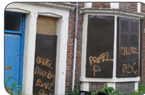
Boarded up house Armstrong street
